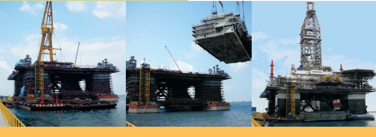
ENSCO 8500, the first of four ENSCO 8500 Series® ultra-deepwater semisubmersibles is under construction in Singapore. Delivery is expected in the third quarter of this year.
